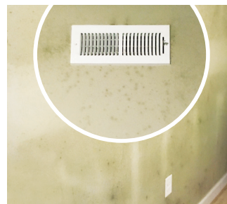
Microbial growth on the walls prior to the installation of an Ultra-Aire MD33 In-Wall Dehumidifier.
