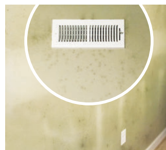
Microbial growth on the walls prior to the installation of an Ultra-Aire MD33 In-Wall Dehumidifier.
